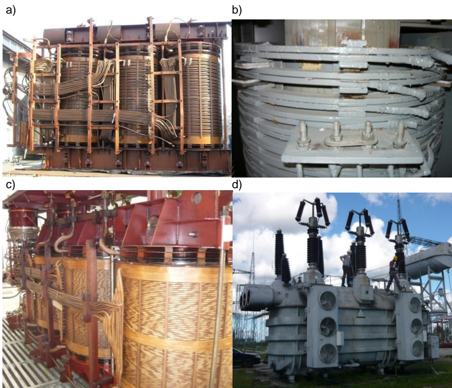
Fig. 1. Transformers used for deformational tests: a) active part of unit A, b) winding with axial deformation of unit B, c) active part of unit C, d) autotransformer D.
